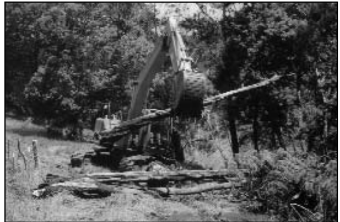
Logs were used to block cows as old fence was removed and new was installed.
